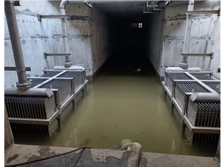
Figure 8. Heat exchanger at tailrace
