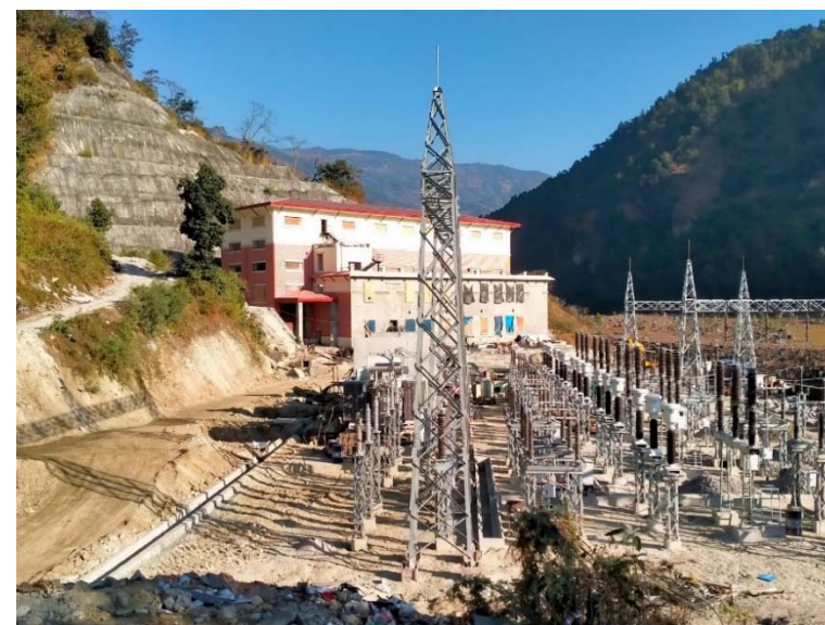
Figure 7. Switchyard and powerhouse view
