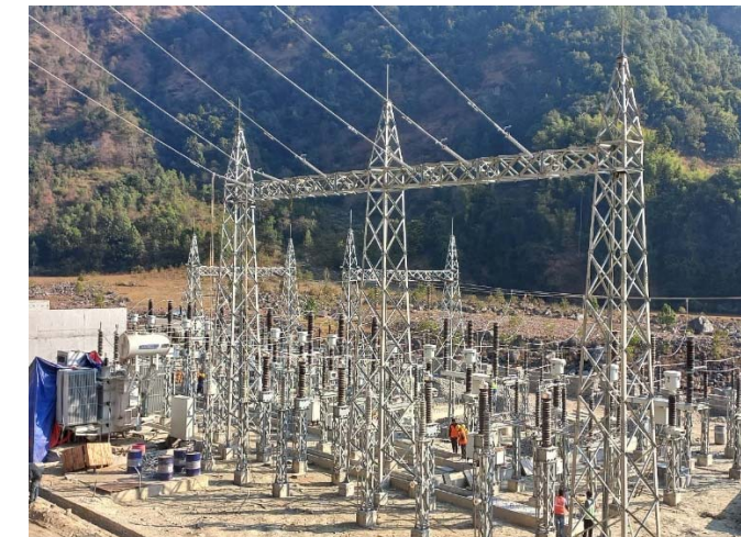
Figure 6. Switchyard nearly ready for testing and charging
