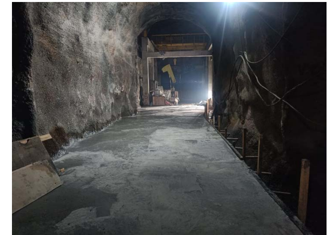
Figure 3. Valve chamber area
